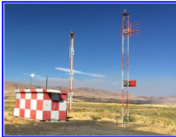
(a) LAMS installed at KDLS.
