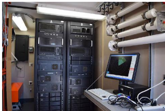
(b) Interior of a LAMS unit.
