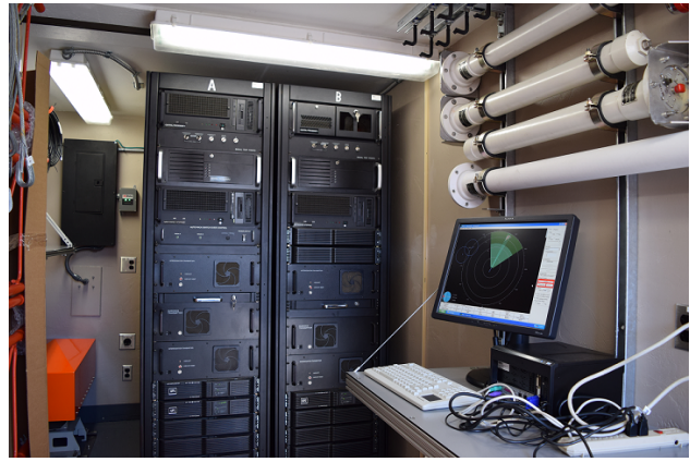
(b) Interior of a LAMS unit.
