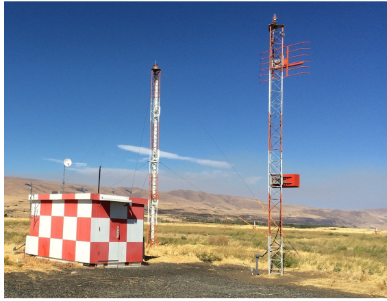
(a) LAMS installed at KDLS.
